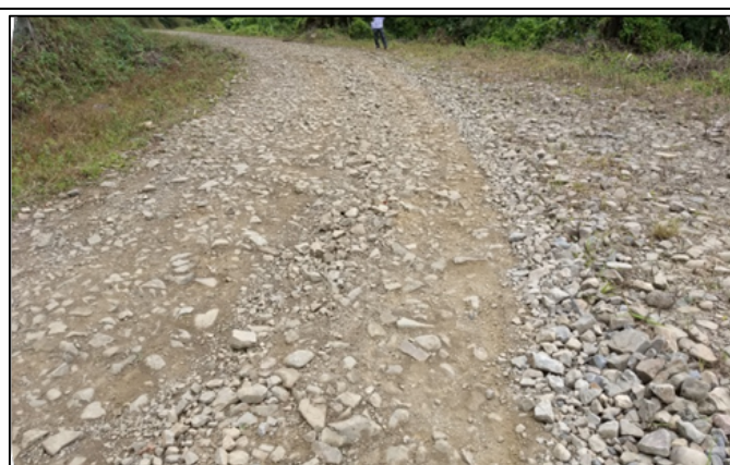
Poor Condition of Pavement
